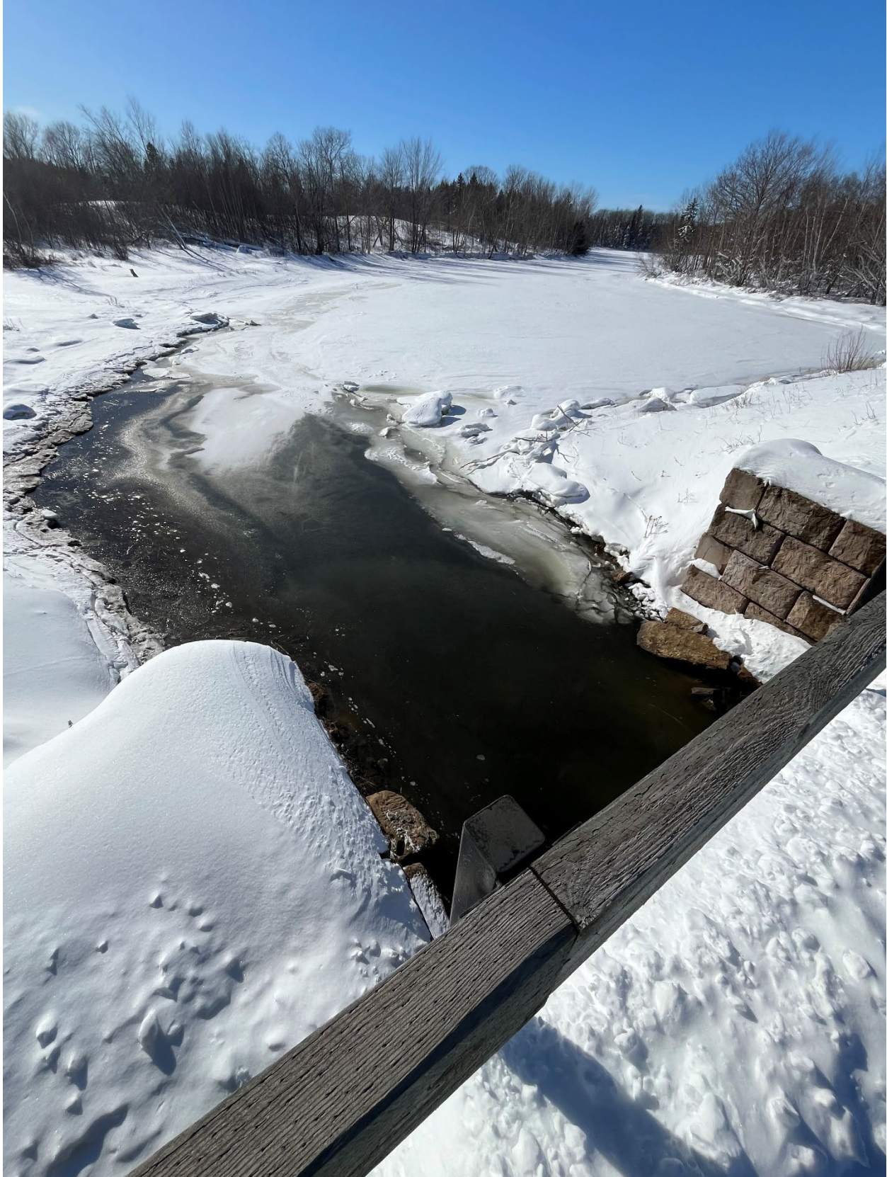
Figure B-9: MacLean Lane bridge showing one of two tidal inlets from Big Gut
